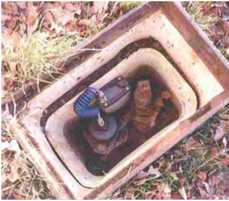
Typical pressure logger installation with hydrant cap and flexible hose
