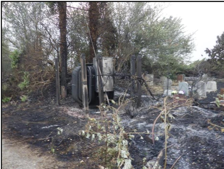
Image 4: Electrical substation – near to Church
