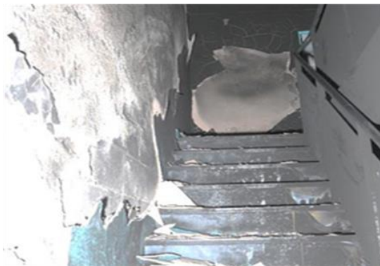
Image to left: View upstairs showing extensive heat and smoke damage.
