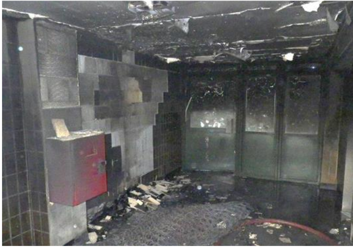
Image left: View of communal area with the remains of the mattress in foreground. Note damage to ceiling and walls, doors and wall panels.
