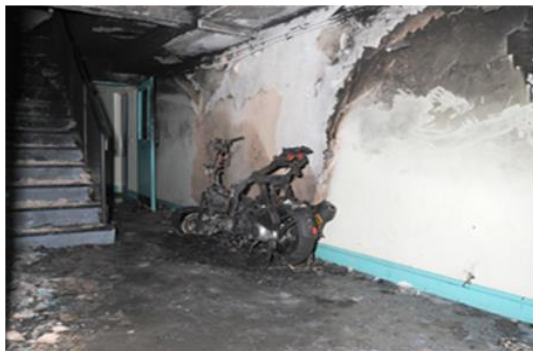
Clear burn pattern behind the scooter Note: rear tyre is still intact
