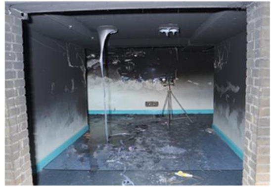
View going in through the communal entrance. Note light fittings have melted
